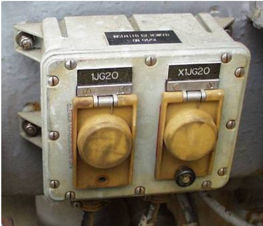
Glenair Modar Electrical Box on DDG-52, 2003
