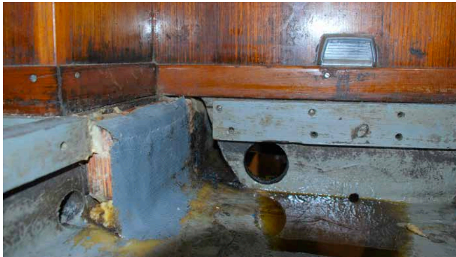
Inadequate tabbing detail
