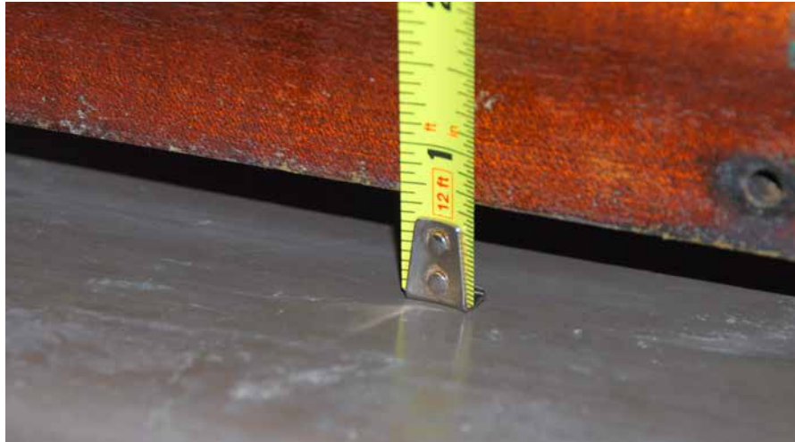
Bulkhead separated from stiffener
