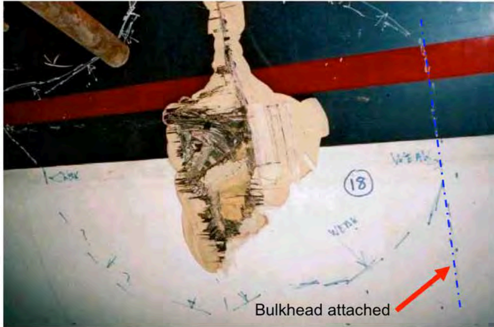
Full extent of impact damage to hull sandwich construction [Laser Technology, Inc.]
