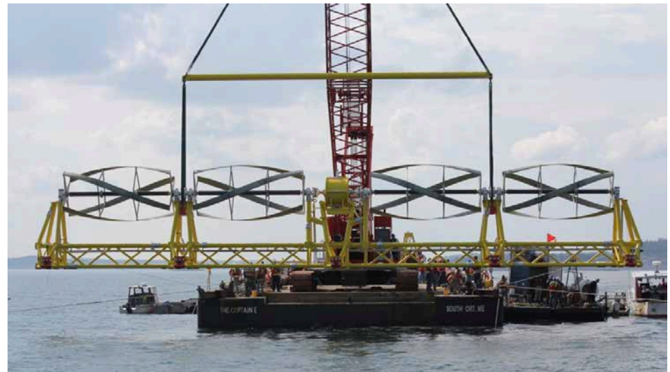
ORPC installed the country's first grid-connected, Commercial TidGen™ Power System at a 60-acre site in Cobscook Bay, Maine
