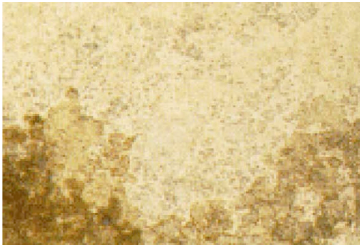
Dry Spots Area of reinforcement that was not wetted with resin. Usually at laminate edge.
