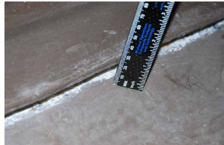
Failed Grid Stringer Installation
