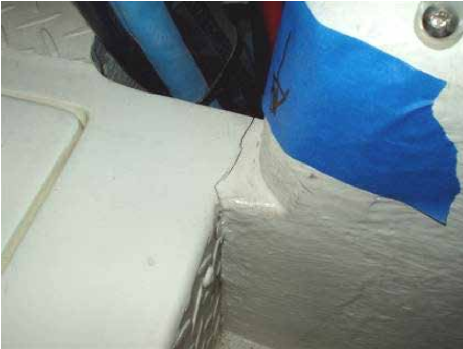
Engine girder cracking apparently from improper hauling sling arrangement
