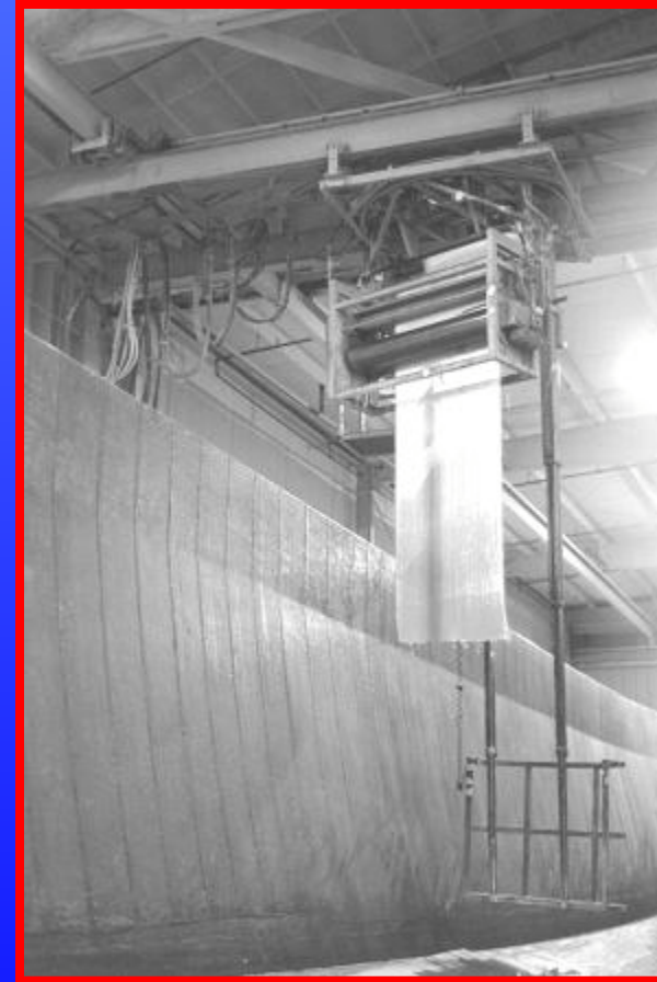
Impregnator on Overhead Gantry for Open Molding of Large Hulls at Westport Shipyard
