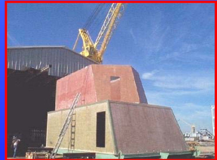
MARITECH Composite Superstructure Project Built by Structural Composites and Ingalls using Adhesive Technology
