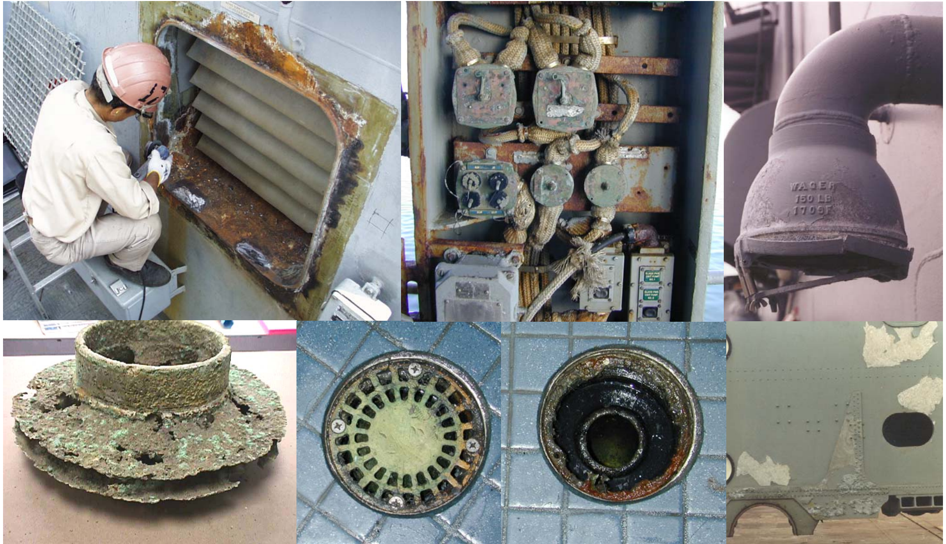
Examples of Corroded Metal Components on Navy Ships [Jeff Goldring, NAVSEA 05M3 & Author]
