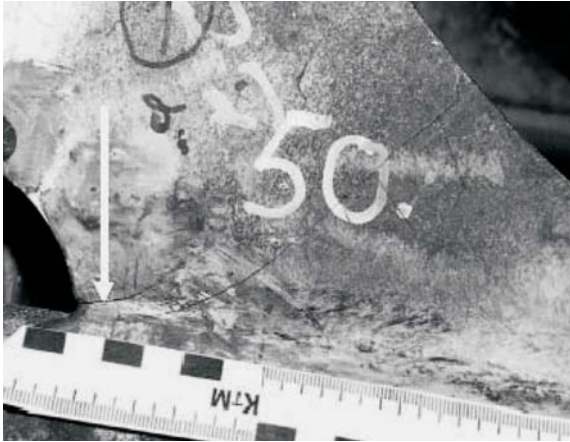
Figure 3. Fatigue Crack Initiated at Bilge Web Detected by Piezo Gauges [ref 8]
