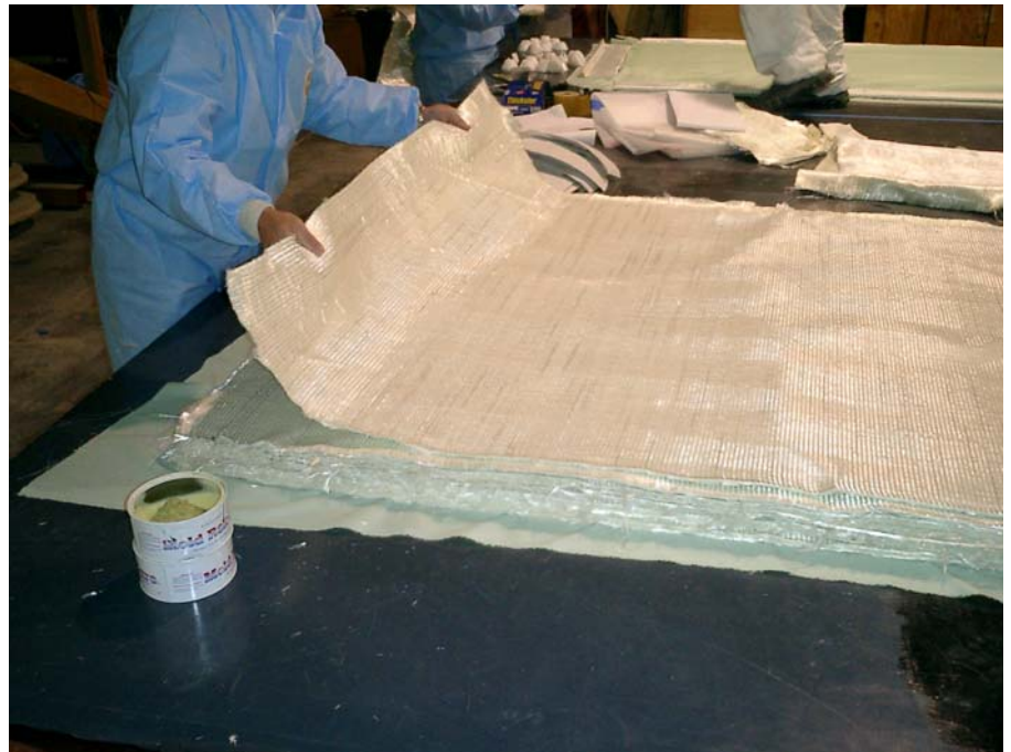
Figure 1. VectorFusion™ E-3LTi 10800 x 21 layers being prepared for infusion. In this case, the finished part is a thick component at a hydro power site. (photo courtesy of Vectorply Corporation)
