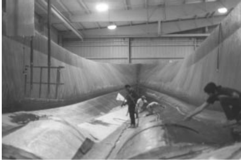
Figure 5-30 Laminators Consolidate Reinforcement Material Applied by Impregnator at Westport Shipyard [author photo]
