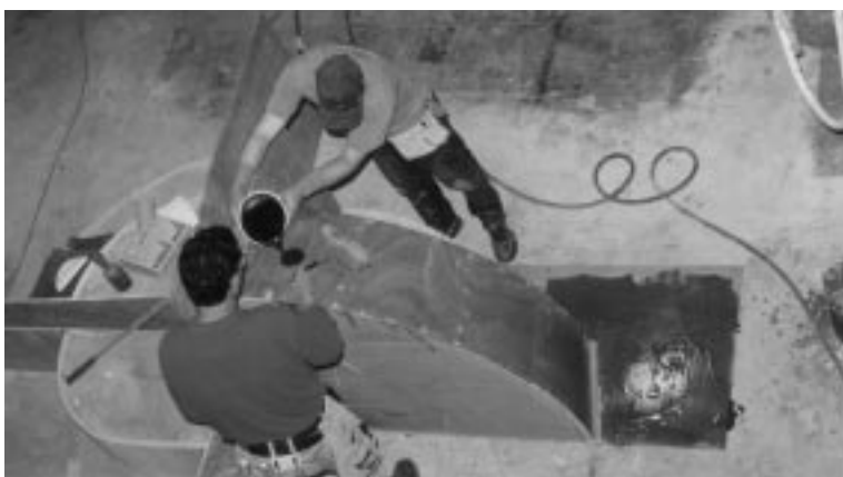
Figure 5-17 Resin is Applied to a Plywood Form at Heisley Marine [author photo]
