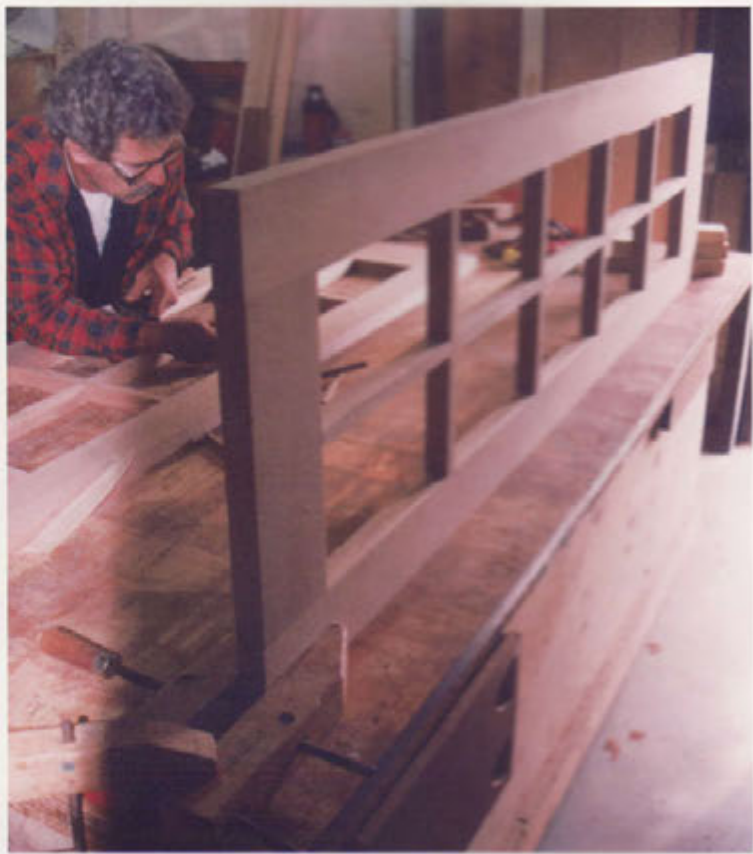
Carpenter Ron Wiren works on French doors that separate the den and dining areas.
